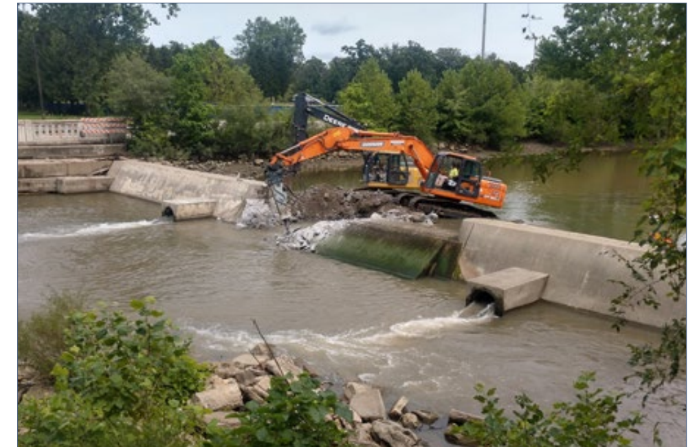
FIGURE 2.8-38 | The formerly clogged spillway pipes were cleared prior to removing the center of the dam.
