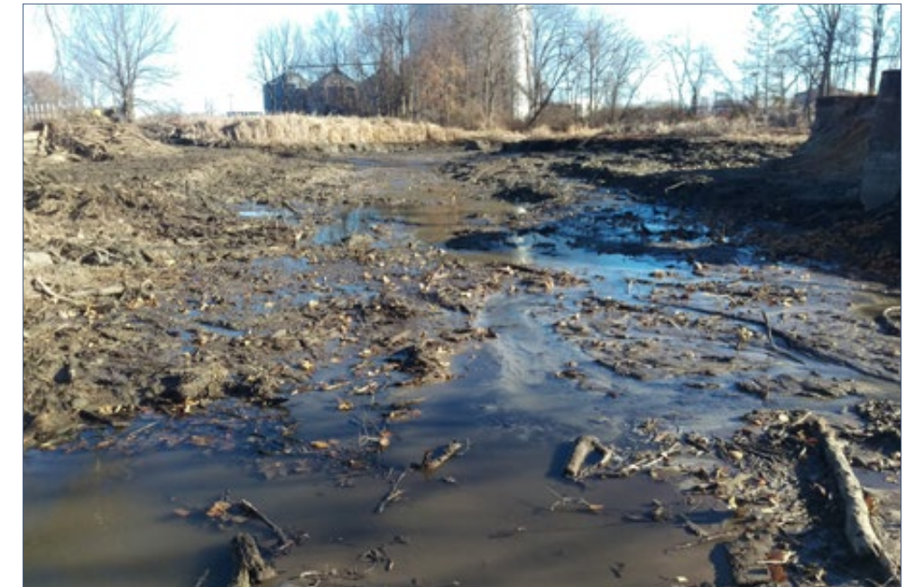
FIGURE 2.8-22 | A check dam was used to dewater the dam's backwater as the earthen portion of the dam was removed.
