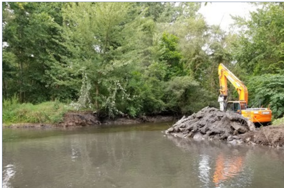
FIGURE 2.8-27 | Concrete and rebar is piled next to former dam location following removal. August 14, 2018.
