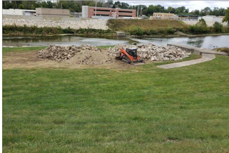
FIGURE 2.8-41 | Boulders are piled near dam prior to modification. October 3, 2019.
