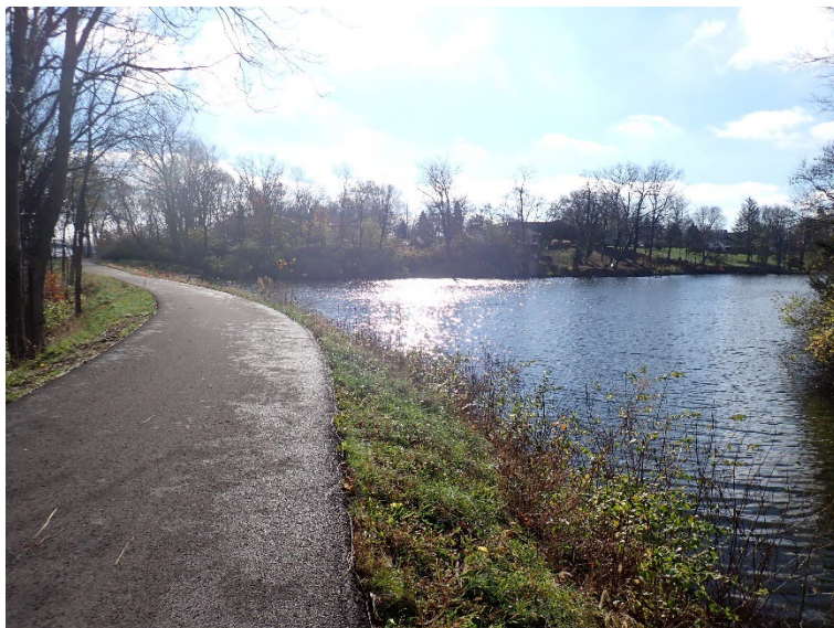
2. A view of the upstream slope at the left end of the dam. Note the heavy brush.
