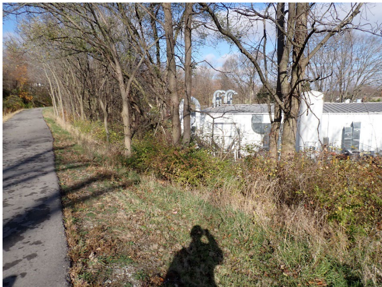
6. A view of the downstream slope at the right end of the dam. Note the trees and heavy brush.
