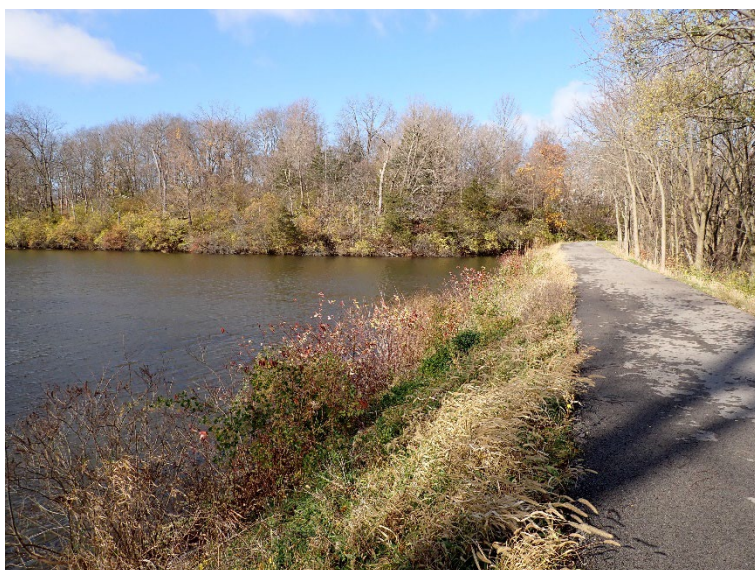
3. A view of the upstream slope at the right end of the dam. Note the heavy brush.
