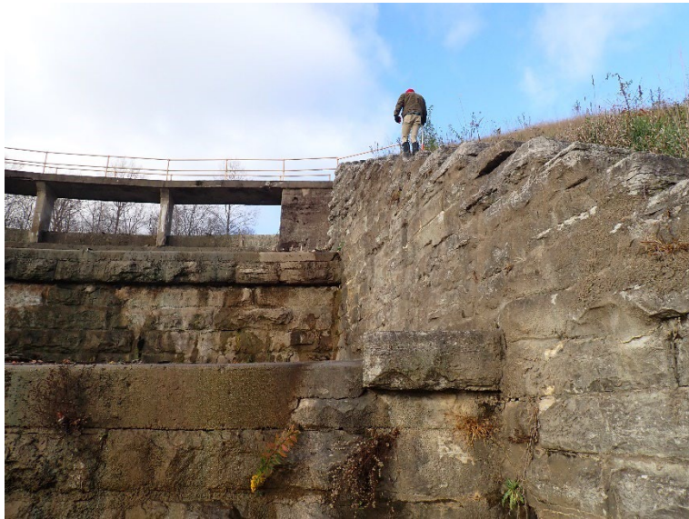
13. Left sidewall of spillway #2. Note the stone is deteriorating and vegetation growing between the joints.
