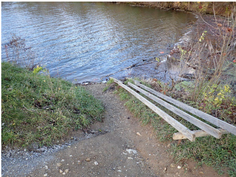
5. Erosion of the upstream slope near the left end of the dam.
