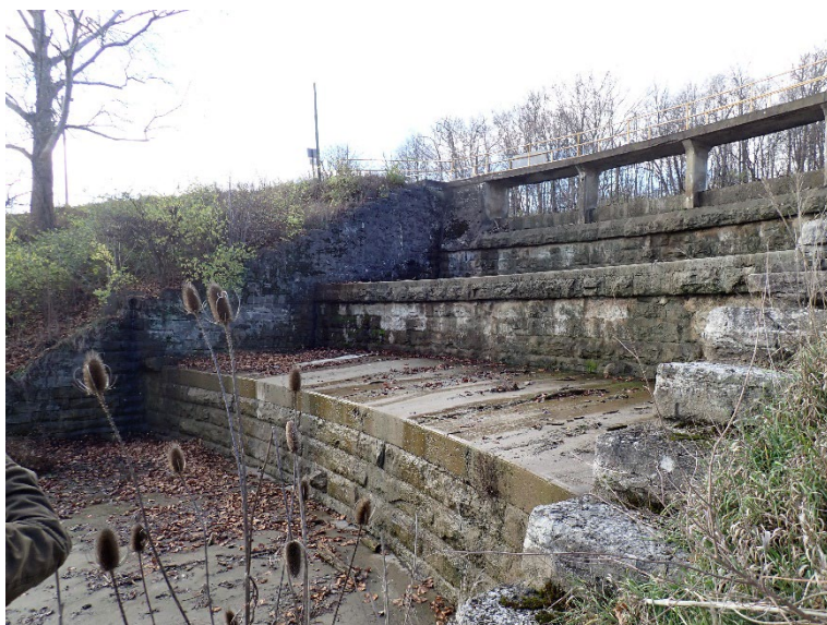
12. Spillway #2 outlet. Note the seepage through the joints.
