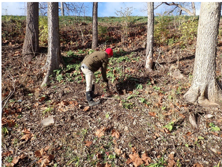
9. A view of a rodent burrow identified on the downstream slope.
