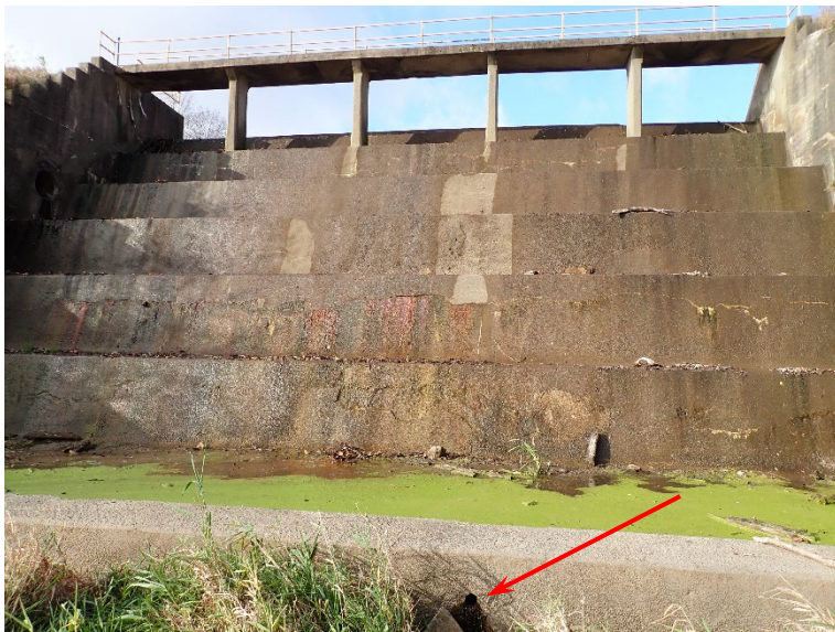
23. View of spillway #3 outlet steps and stilling basin. Note the delamination of the concrete on the steps. Arrow points to a drain for the stilling basin.
