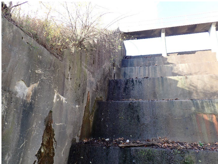
20. Right sidewall of spillway #3. Note the deterioration, efflorescence, and seepage.
