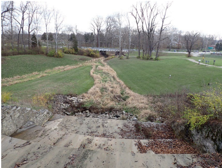
16. Outlet channel downstream of spillway #2 (center). The channel on left side of this photo is the outlet channel for spillway #3.
