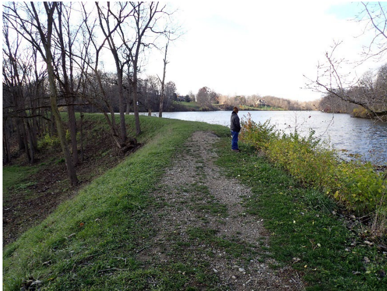
7. Crest at the left end of dam. Note the large bare area.
