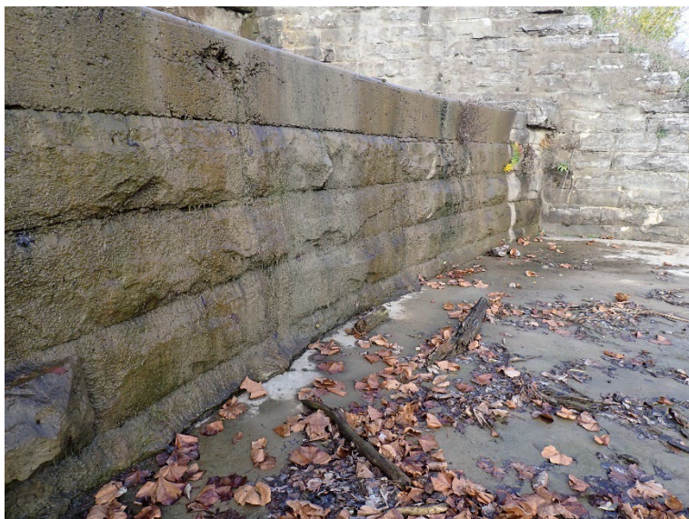
15. Although Spillway #2 was not flowing, the stepped faces of the outlet were wet.
