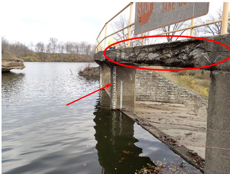
11. Inlet to spillway #2. Note the severe deterioration of the concrete (circled) and the location of the staff gauge (arrow).
