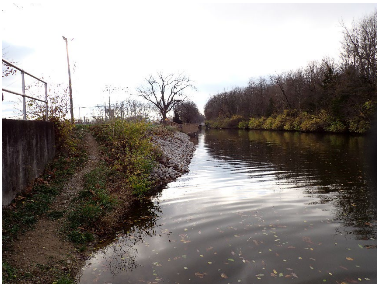
2. Upstream slope adjacent to the right sidewall of spillway #2. Note the erosion and lack of vegetal cover.
