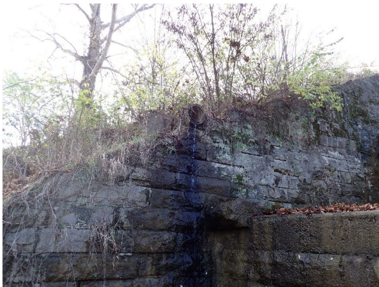
14. A surface drain discharging over the right sidewall of spillway #2.
