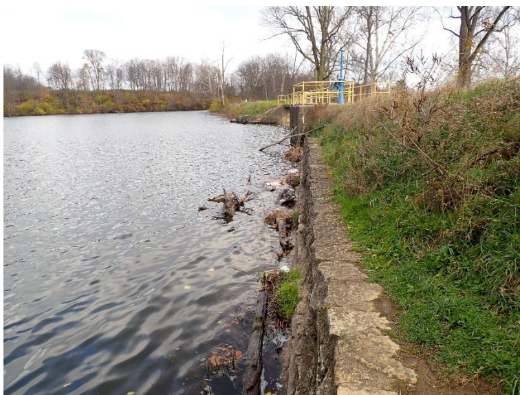
3. Retaining wall and upstream slope between spillway #2 and #3. The vegetation on the slope is too tall.
