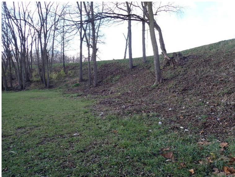
8. Large bare areas on the downstream slope near the left end of the dam. Also note the trees.
