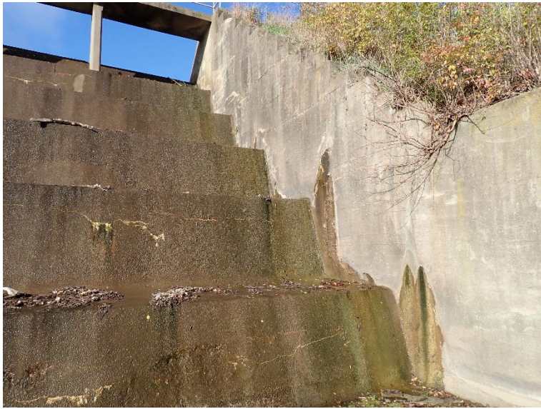
22. Cracking and seepage through the left sidewall of spillway #3.
