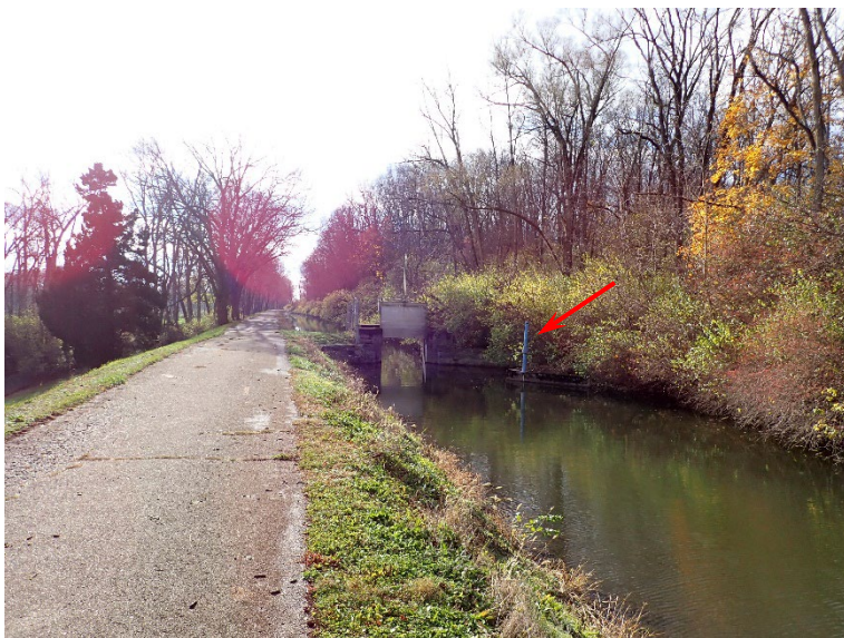
24. Gate to separate the canal from Swift Run Reservoir. Arrow points to a valve control to allow water to bypass gate.
